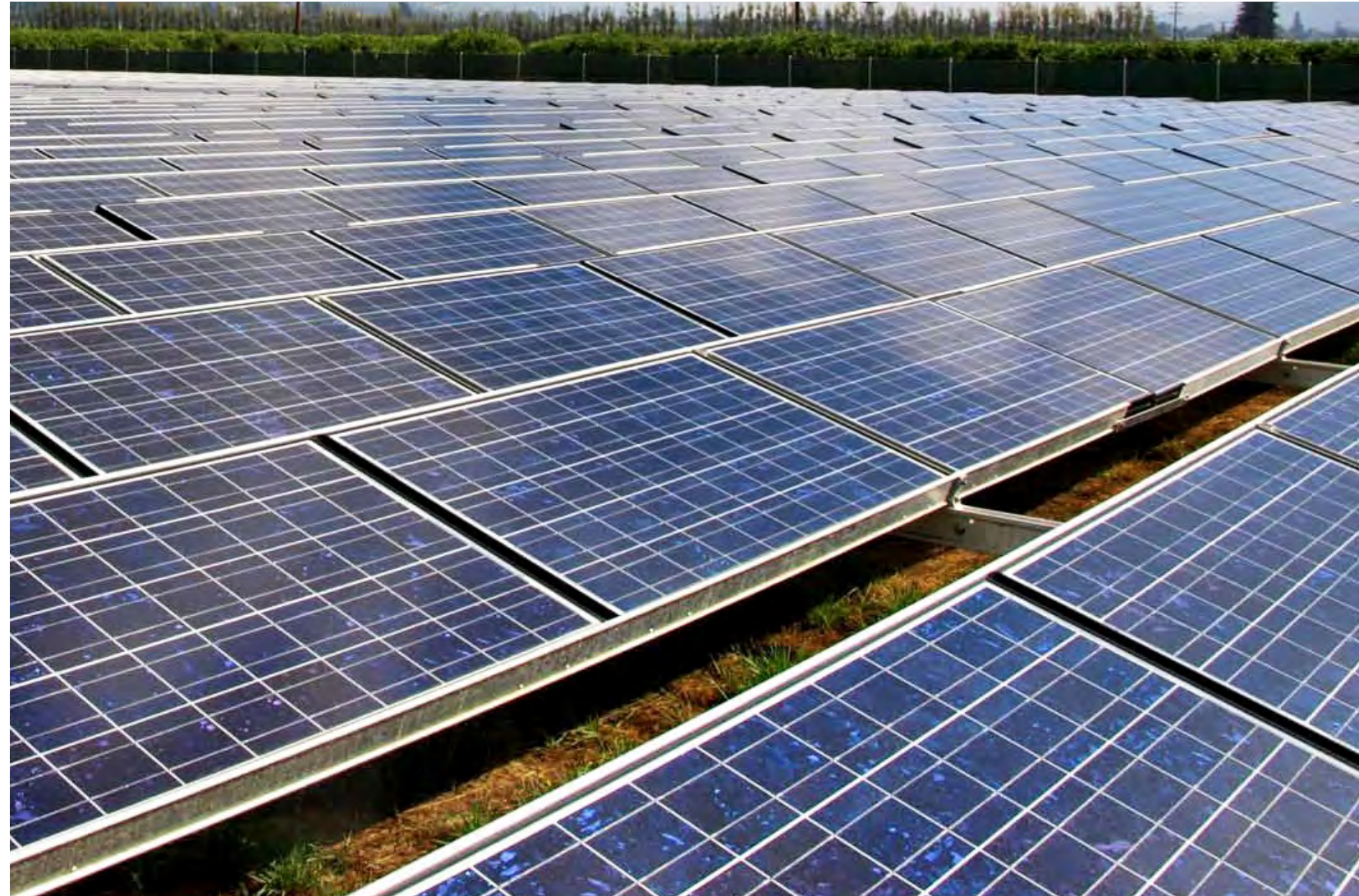
Hunt Companies affiliate Moss built Kalaeloa Solar Park in Honolulu County, Hawai'i. The company is one of the largest self-performing EPCs in the solar market with over 15GWs of experience.
